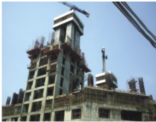
Figure 2. Palas Royale—The Tallest Building in India under construction with M-80 Concrete Columns in Self-compacting Concrete
