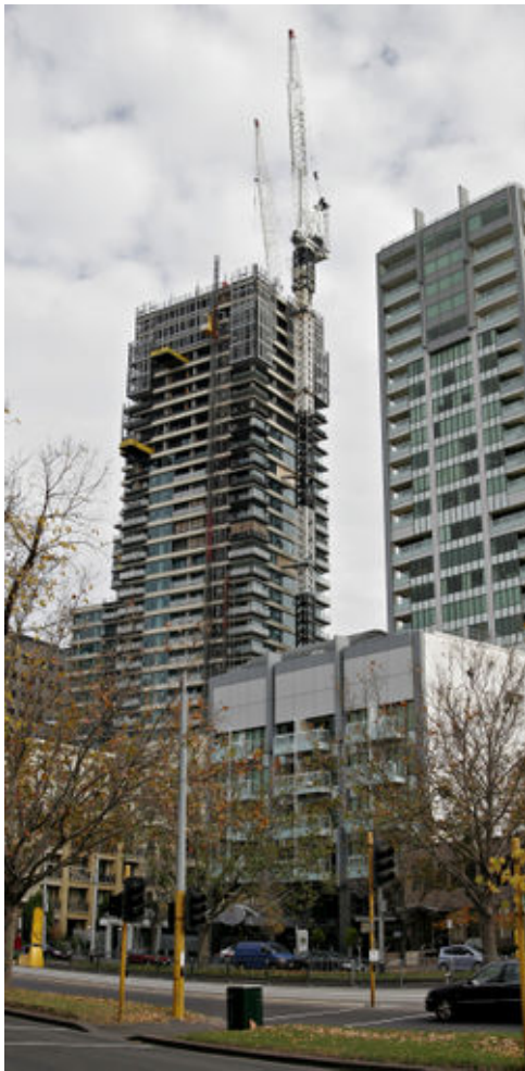
In large construction projects, such as this skyscraper in Melbourne, cranes are essential
